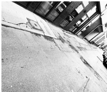
damaged separation of pavements
