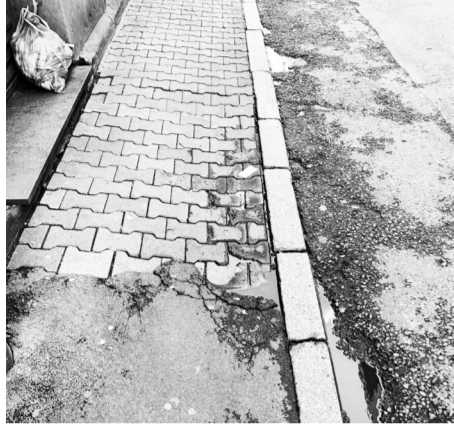
street damage + trash issue
